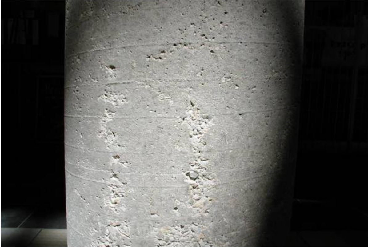
Figure 2: Bug holes and imperfections of a conventionally formed concrete...
