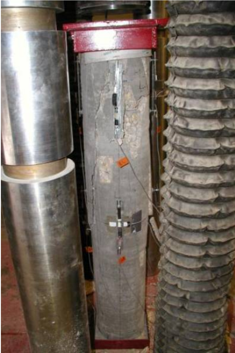
Figure 65: Column FF-FAC after failure.
