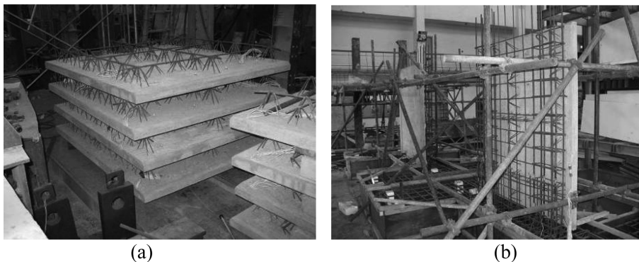
Fig. 2 Manufacturing process of the specimens (a) prefabricated walls, (b) binding process of the steel bars in cast-in-place part
