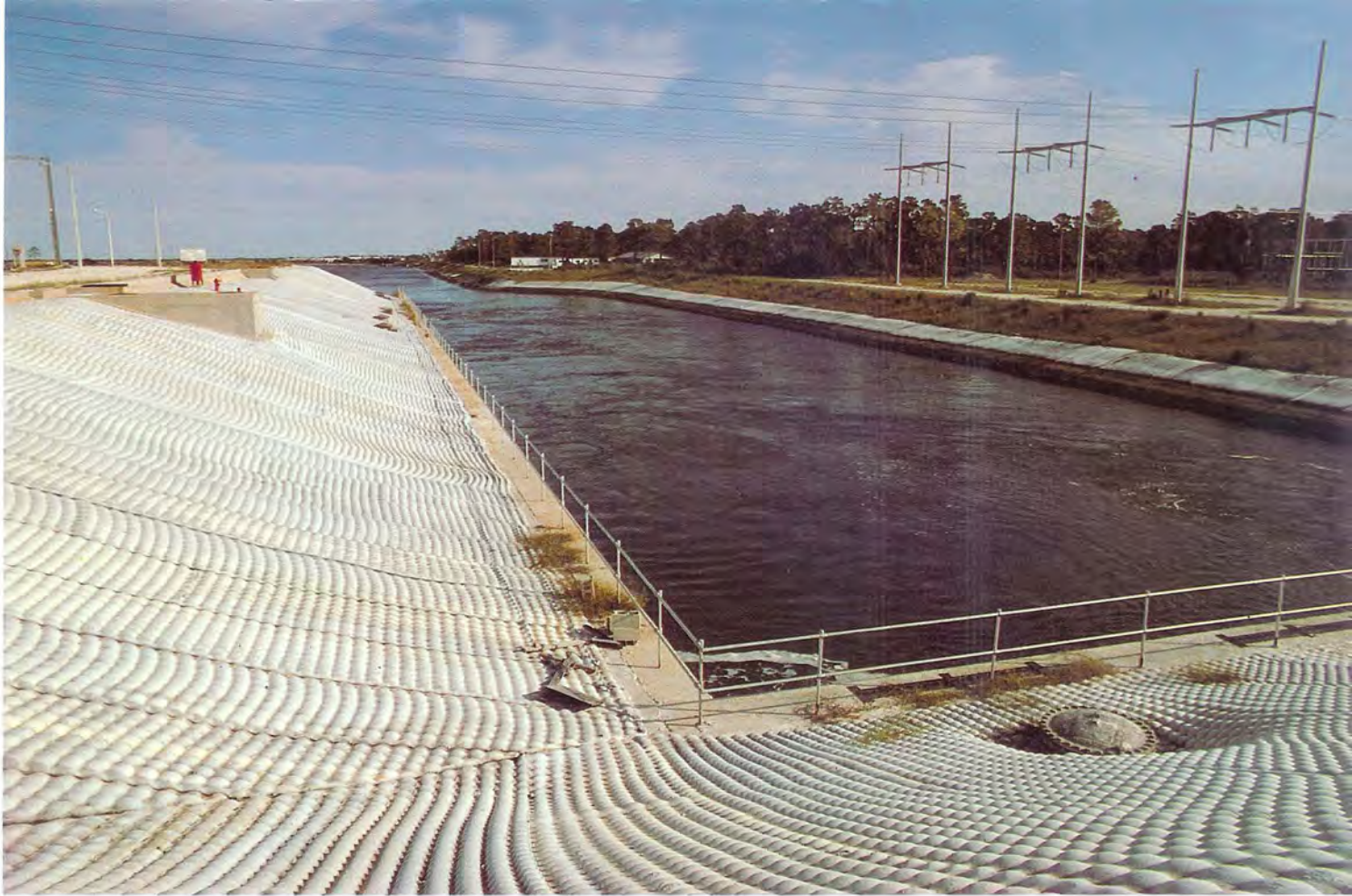
Fabric revetment protects 174,000 square feet 17 of the slope of the discharge canal of the fossil-fueled Anclote plant in Tarpon Springs, Florida owned by Florida Power Corporation.
