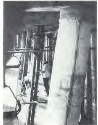
Three men are applying jacket to a pile. In the foreground is a jacketed pile that has been concreted.
