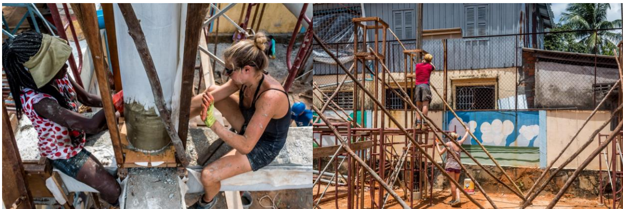
Figure 5a: Column clamped at base during first pour Figure 5b: Column falsework to receive beams
