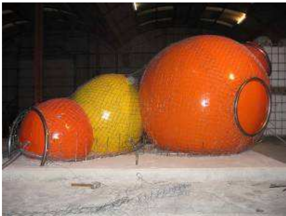
Fig. 15 The balloons covered with wire mesh and the steel rings for the openings.
